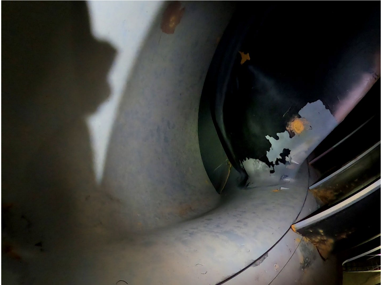
Figure 13.—Blade 7 after 1,000 hours of operation. The PE2 failed by cavitation and delamination on leading edge with approximately 10 square feet of damage. The rust spot near the center of the blade is from the welded brace that was removed for the platform and repaired using an unknown procedure.
