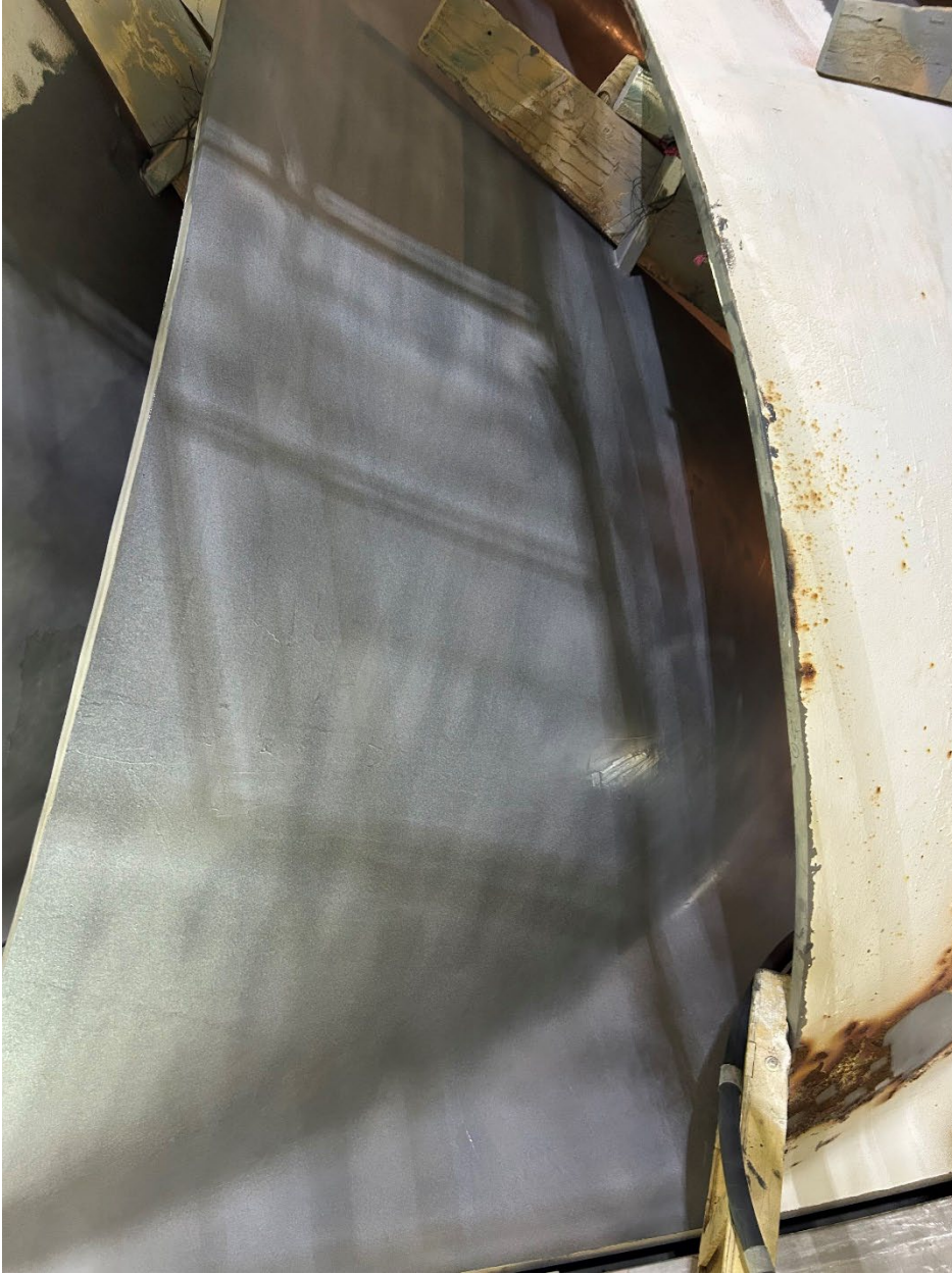
Figure 2.—The surface of Blade 13 primed with ceramic-filled epoxy, shown after sweep blasting.
