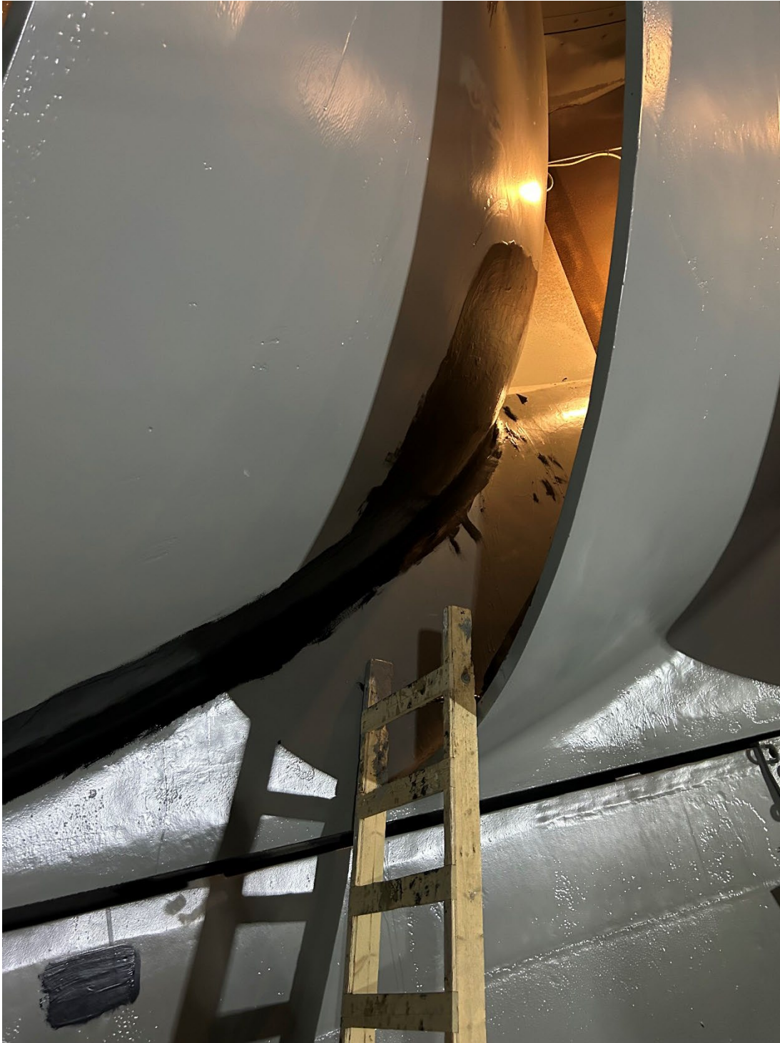
Figure 9.—The cavitation zone of Blade 8 shown coated with solvent-borne epoxy and PE2.
