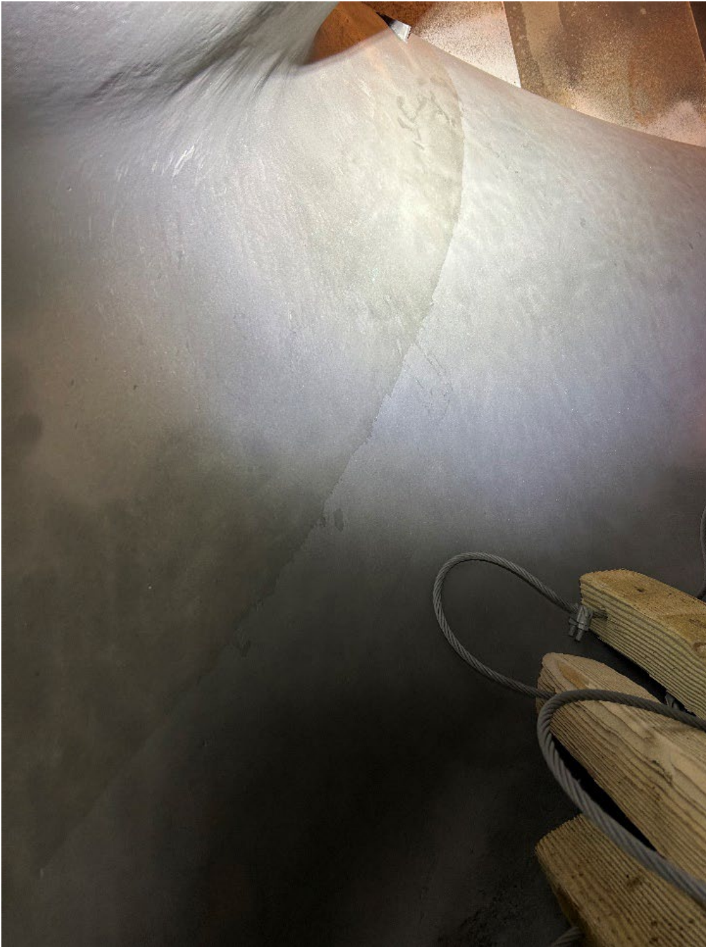
Figure 1.—Typical condition of surface preparation at 308 stainless steel weld overlay/mild steel transition.
