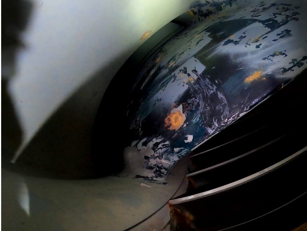
Figure 12.—Cavitation damage on leading edge suction side of PE1, approximately 1 square foot of damage. The gray color is from application defects that were repaired with an epoxy.
