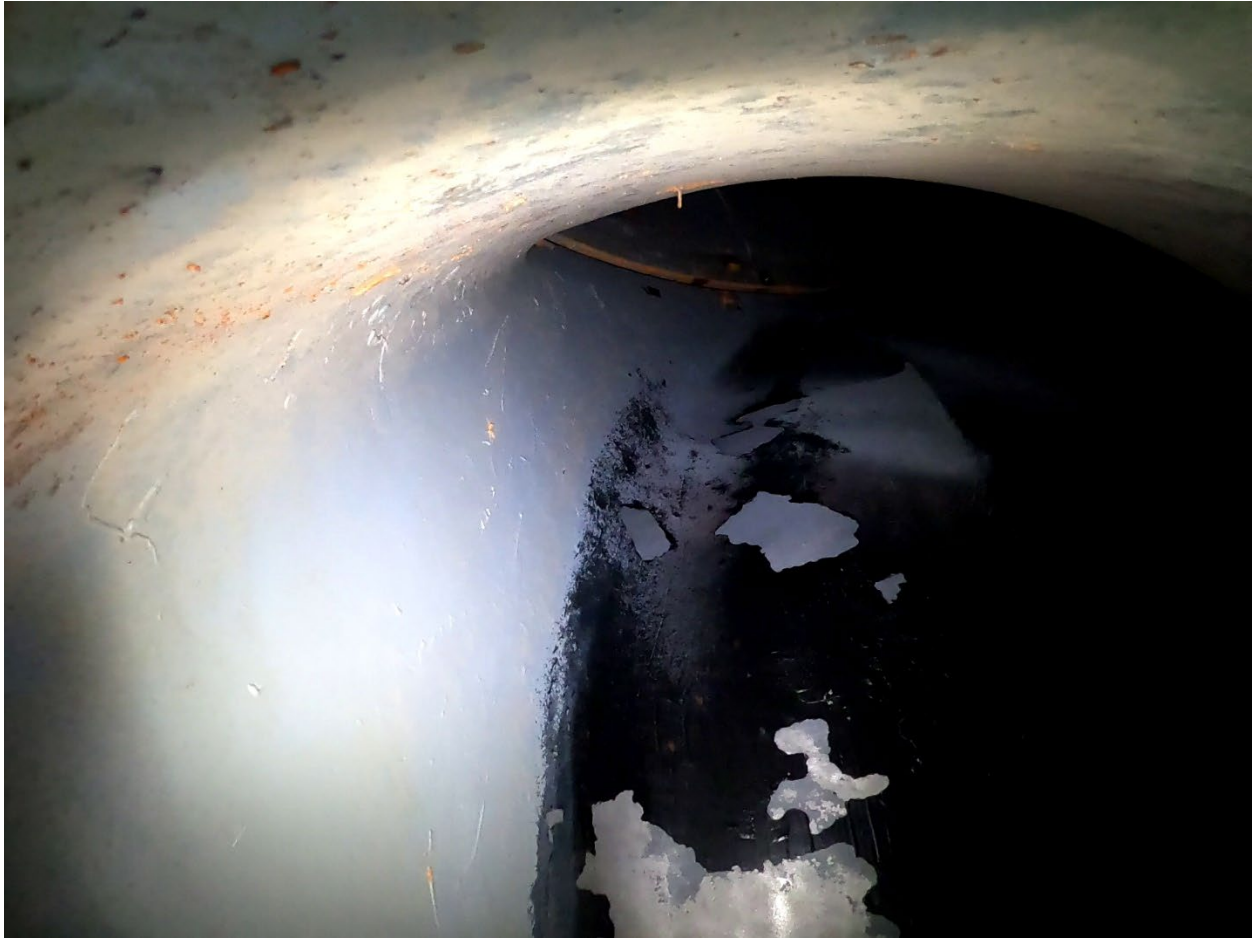
Figure 16.—Close-up of Blade 7 after 1,000 hours of operation. The PE2 failed by cavitation and delamination.
