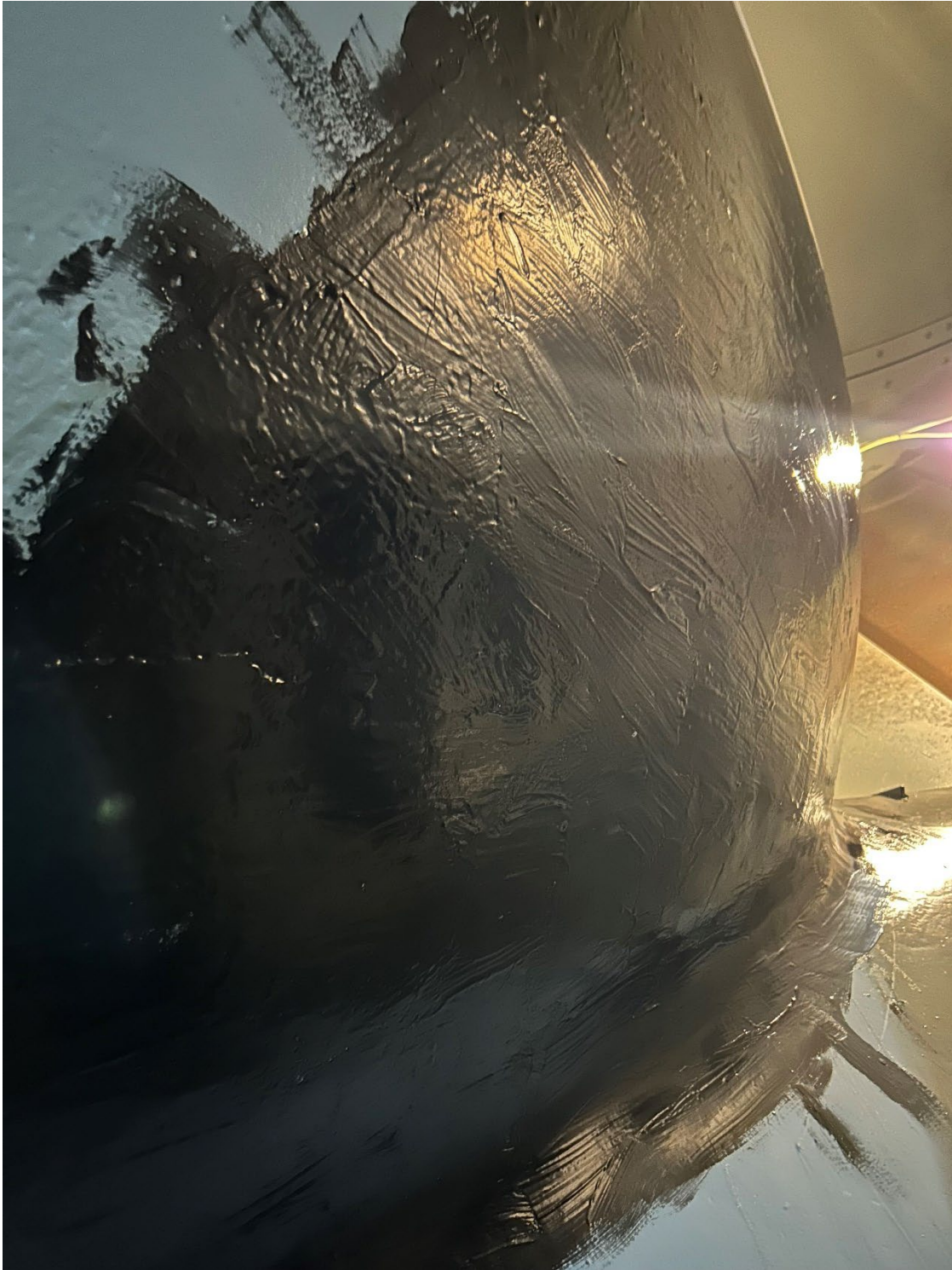
Figure 10.—The cavitation zone of Blade 8 shown coated with solvent-borne epoxy and PE2.
